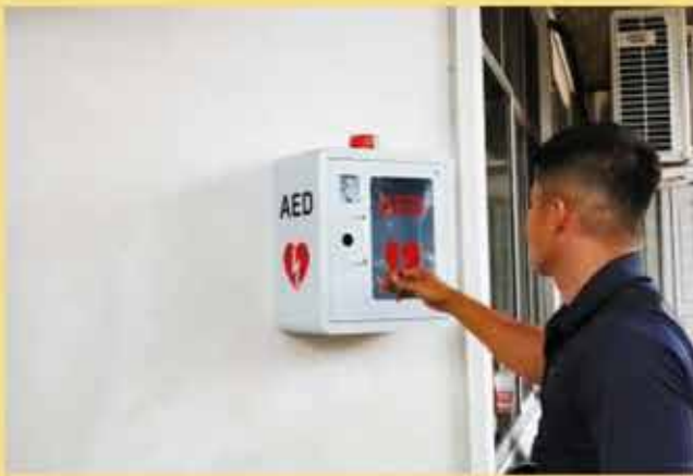
AED installed at Kuching Waterfront Management Office
